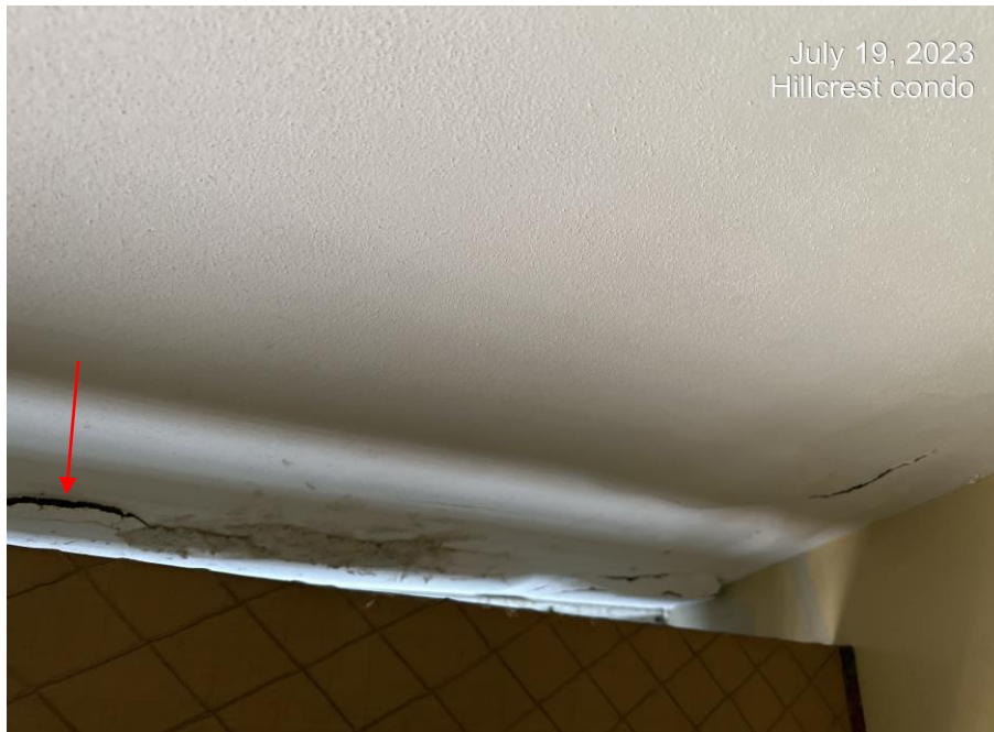
Photo 6: Spalled concrete in the overhead slab.
