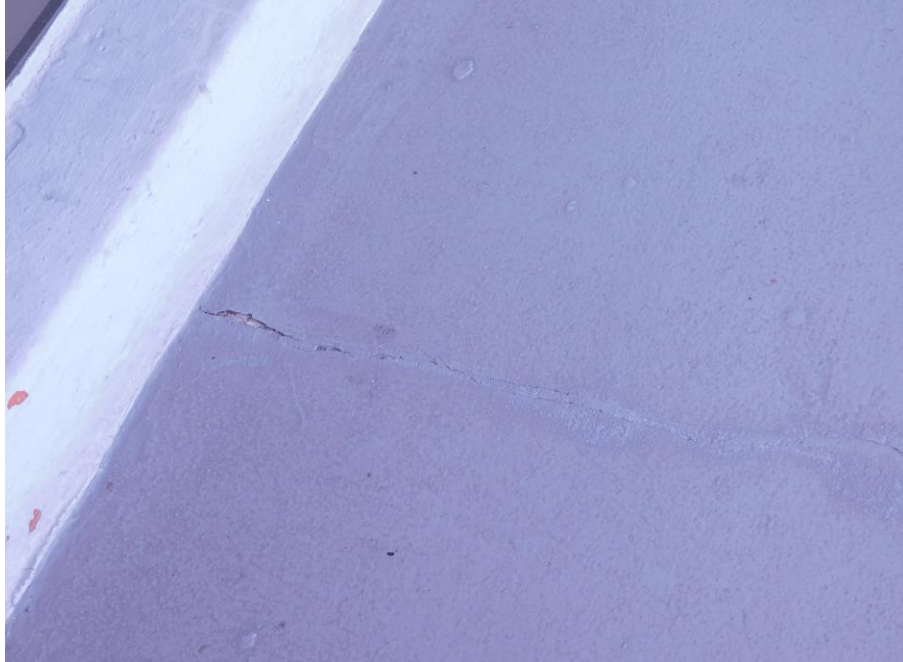
Photo 15: Cracks on the slab in the walkway.
