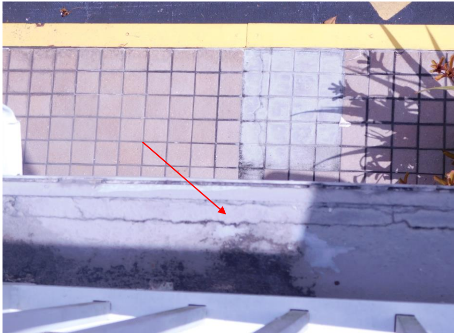
Photo 12: Cracks on the slab edge in the walkway
