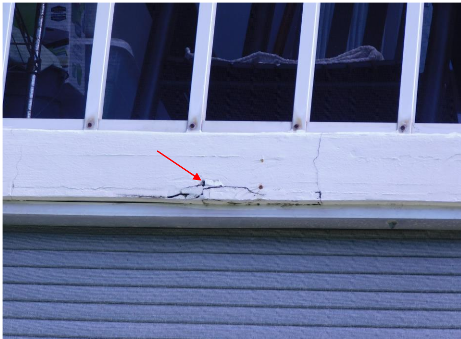
Photo 8: Concrete spalling and cracks on the slab edge.
