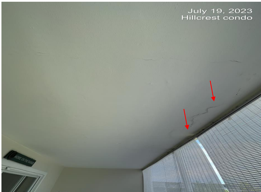
Photo 2: Multiple cracks on the overhead slab.
