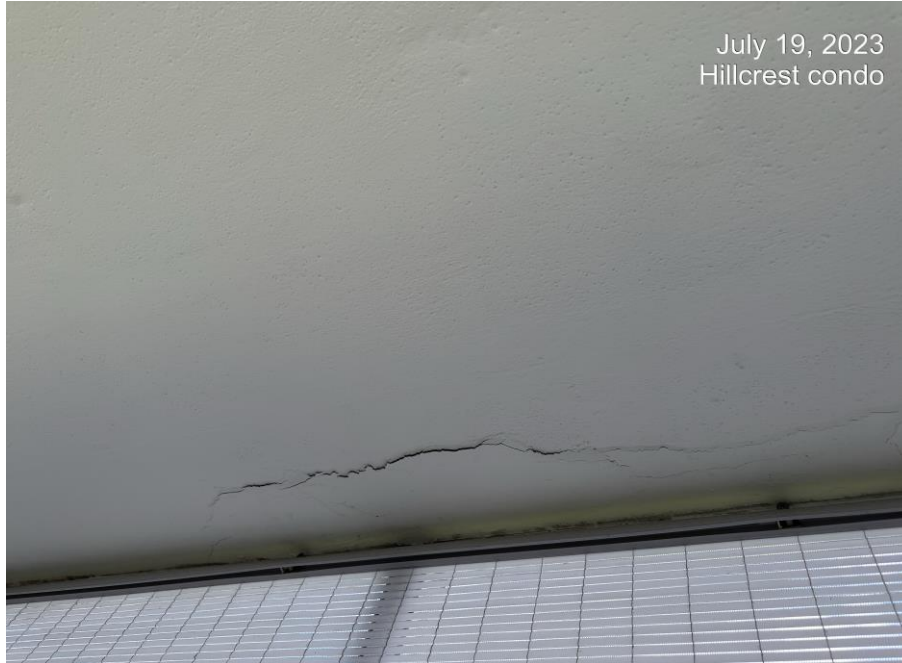
Photo 13: Cracks on the overhead slab in the balcony.
