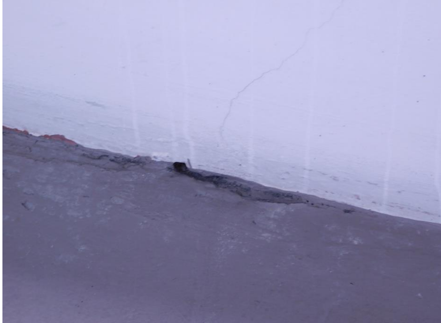
Photo 11: Cracks on the wall in the walkway.
