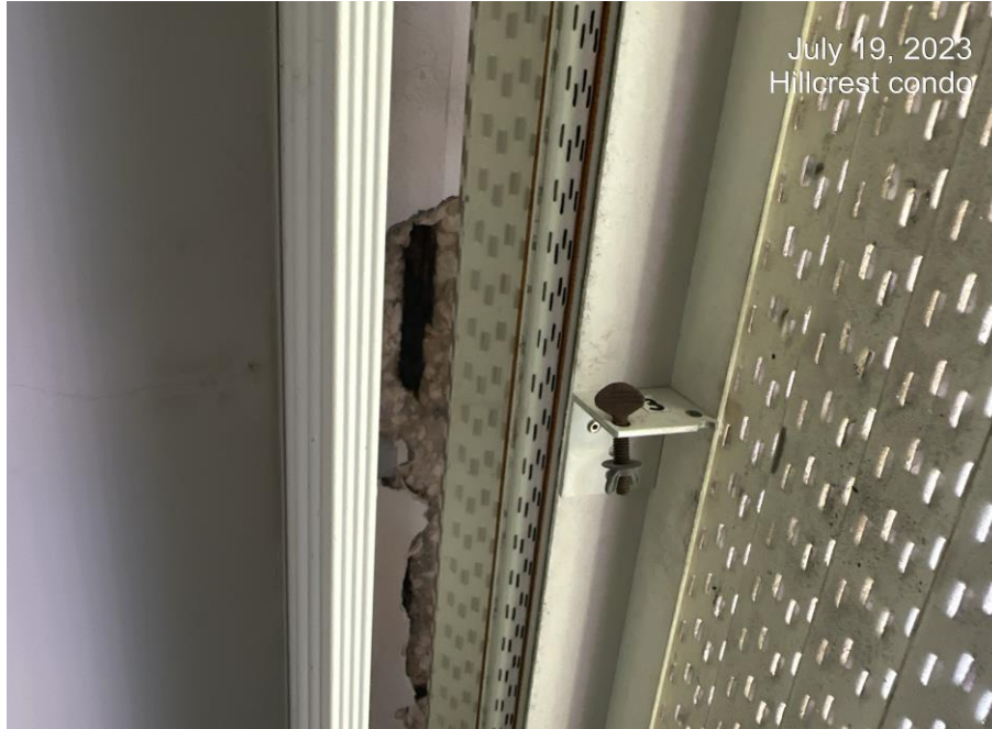
Photo 5: Spalled concrete and exposed corroded rebar in the overhead slab.
