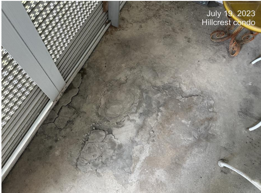
Photo 1: Spalled concrete on the balcony floor slab.
