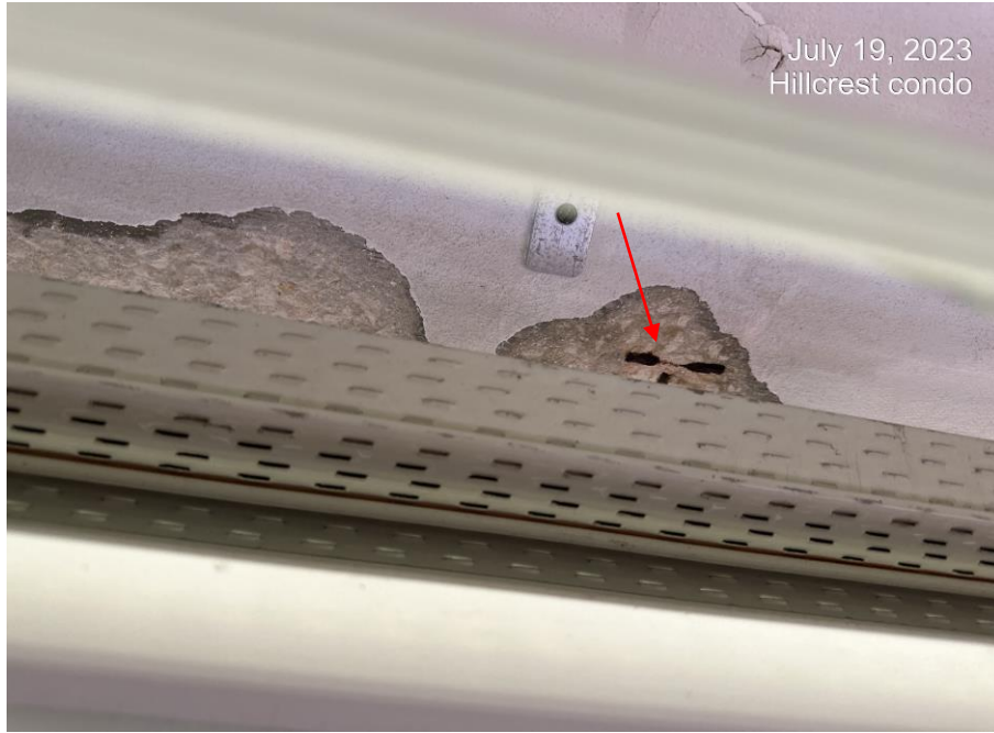
Photo 3: Spalled concrete and exposed corroded rebar in the overhead slab.
