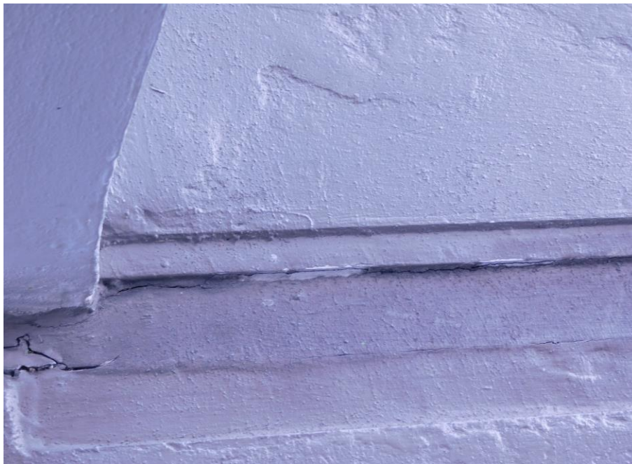
Photo 16: Cracks on the concrete slab in the walkway.
